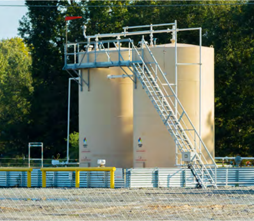
Each production site features secondary containment, such as a berm, to prevent spills from reaching the surrounding environment.
